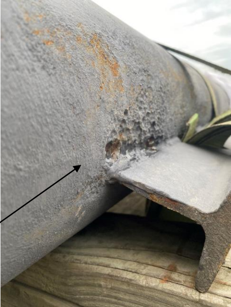
CUI damage on the nearby shoe was found to have greater than anticipated wall loss after blasting and primer coating.
