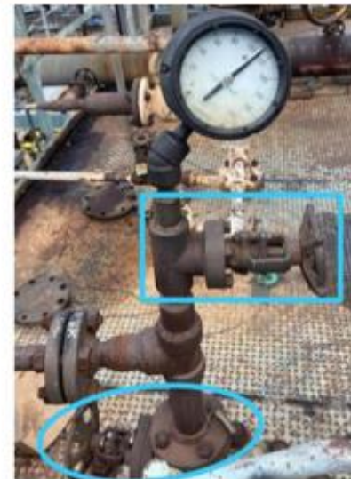
Figure 1. Valves isolating the pressure gauge
