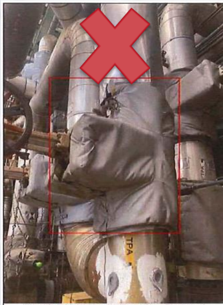
Valve Blanket Installation with Flanged Connection Covered Not Allowed in Services >400^{\circ}\text{F} without Engineering Approval
